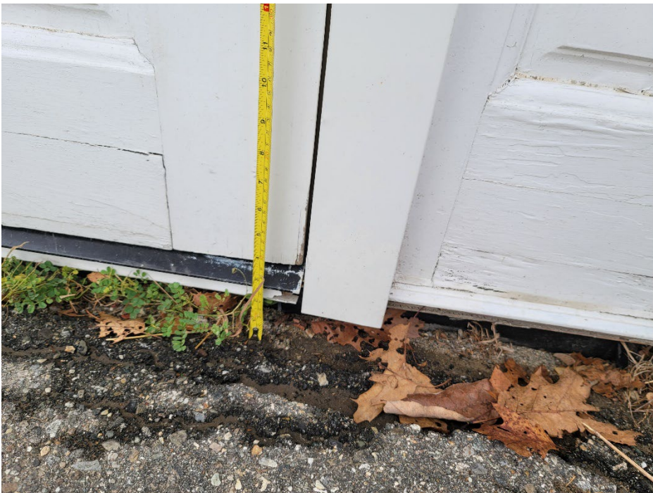
#3: A door threshold of three inches at a marked accessible entrance.
