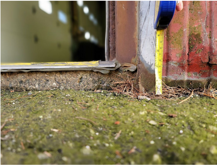
#3: A door threshold of two and a half inches at a marked accessible entrance.
